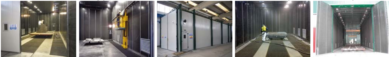
Indoor installation with scrapers and cochlea
